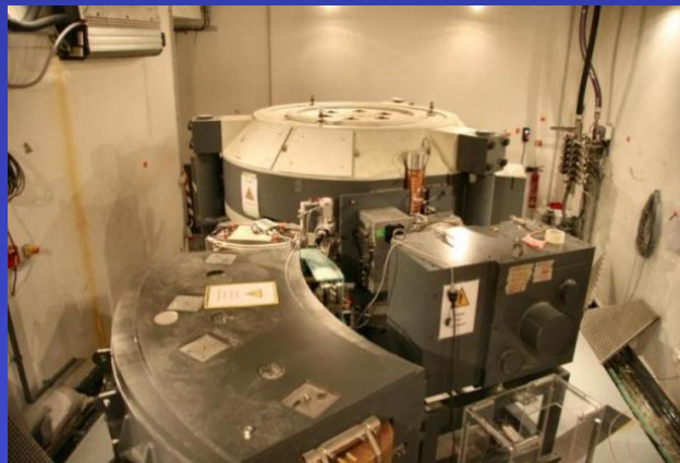
Cyclotron S2C2 (CAL)
