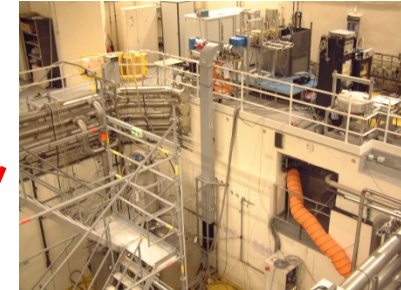
Cryogenic test hall
