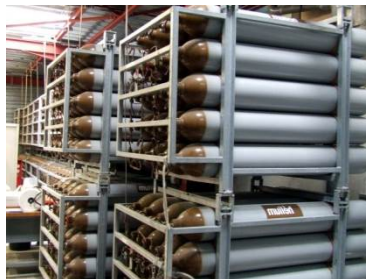
Helium gas recovery & compression
