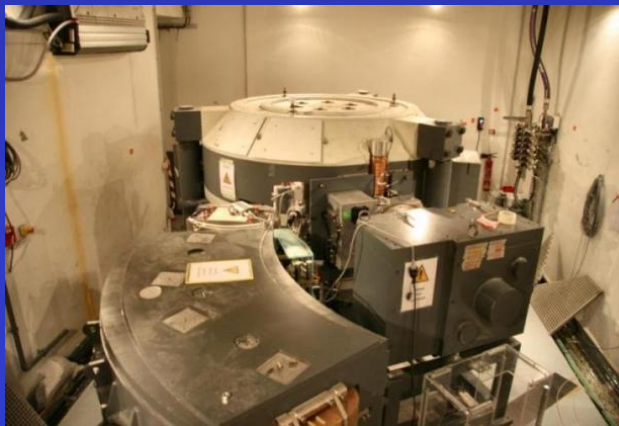
Cyclotron S2C2 (CAL)
