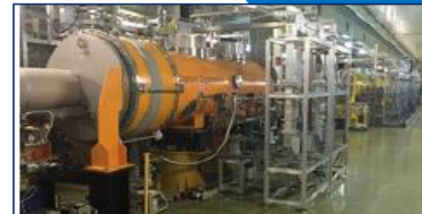
Module test at stF-2
